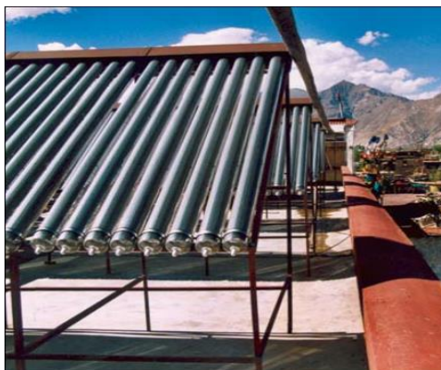
Figure 1.1: Solar panel system
